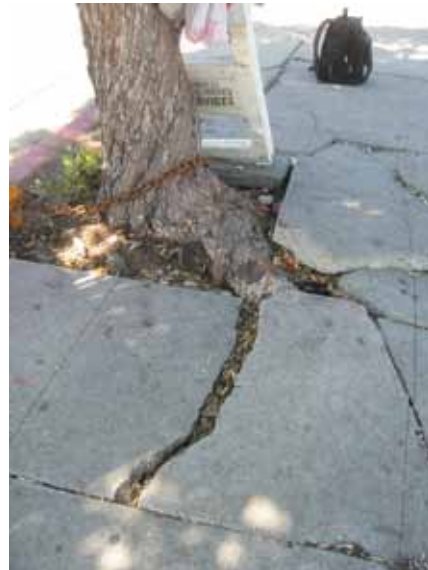
Ficus roots lift sidewalk paving.
