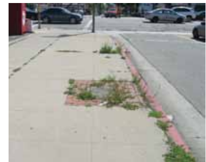
Unmaintained sidewalks have paved-over tree wells and weeds.
