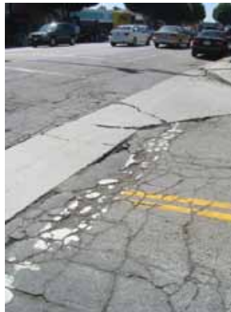
Roadway needs reconstruction.
