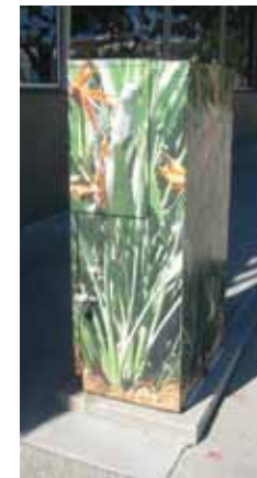
Mural on existing electrical box
