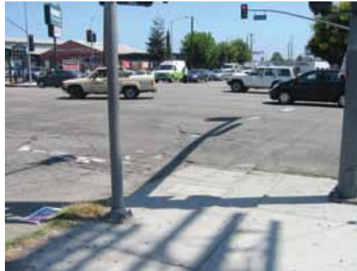
Missing accessible ramps are at the end of the dirt parkway.
